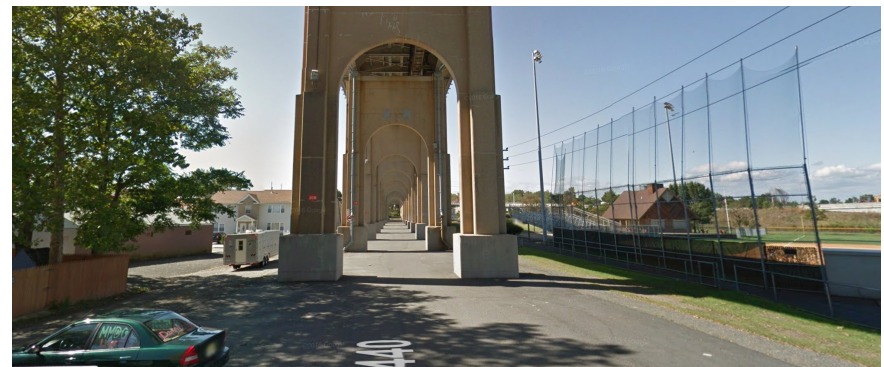
Underbridge Existing Conditions (View from under the NJ-440/Outerbridge Crossing facing State Street)
