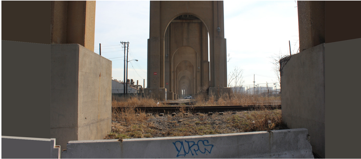
Parker Street Existing Conditions (View looking East Under 440 Bridge Towards High Street)
